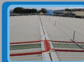
Caution area on the roof of KYB-UMW Malaysia was highlighted with red lines
