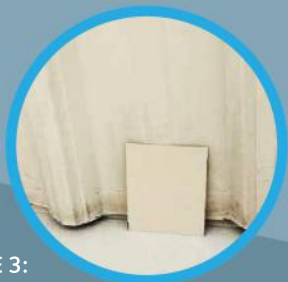
Negligible fading on wall cladding
