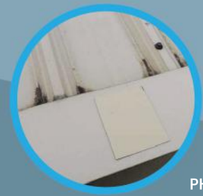
Minor fading on roof flashing
