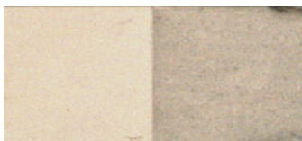
• Discolouration by Dirt Staining
